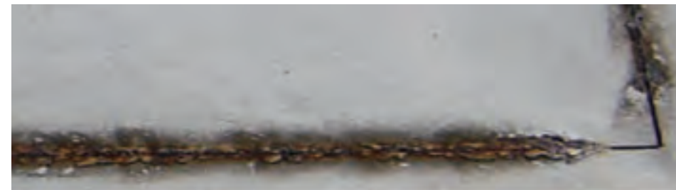
Improper cut example
